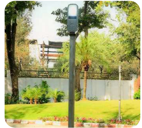
SMART STREET LIGHTS
