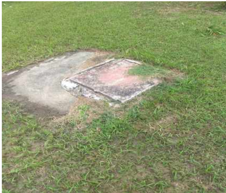
Fig.1. Borewell for ground water recharge
