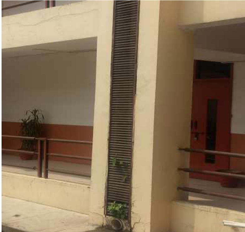
Fig.3. Conduit to carry rainwater from roof to tank.
