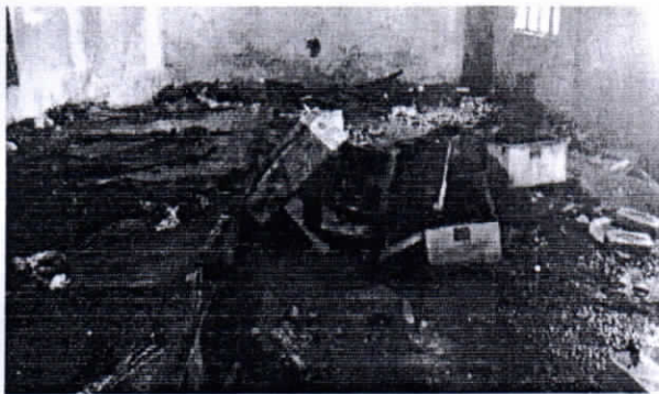
Burn house of Munshi Nagar 12-01-2019
